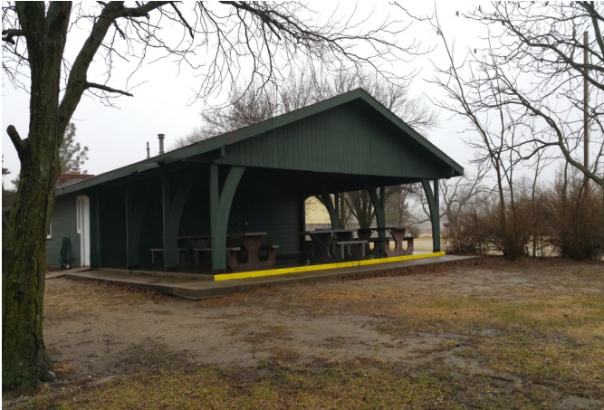
Front View—4 picnic tables and electrical outlets
